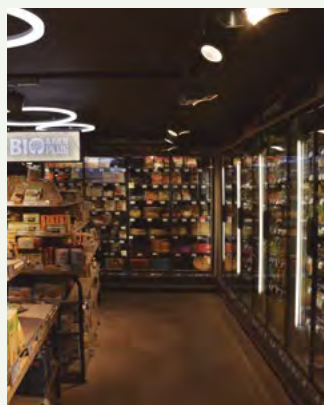
CO 2 installatie in de Carrefour City, La Madeleine. 2 units van 15 kW CO 2 . CO 2
